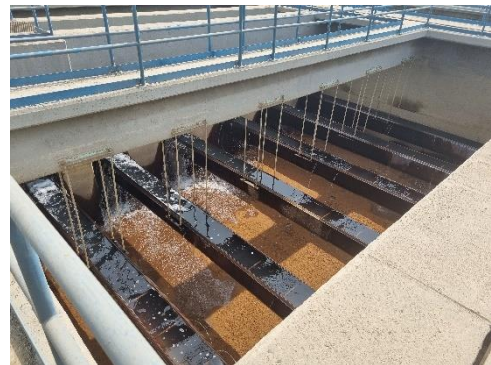
Figure 1 Gravity Sand filter treating river water
